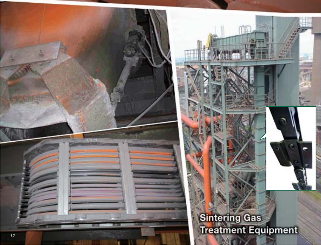
Sintered Ore Apron Conveyor
