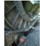
Heavy Duty Roller Chain on a reclaimer drive
