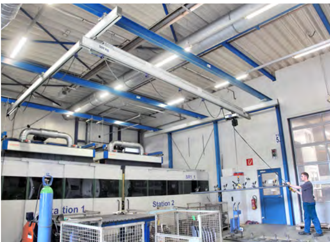
Aluminum single bridge crane system with reinforced section and chain hoist during machine loading
