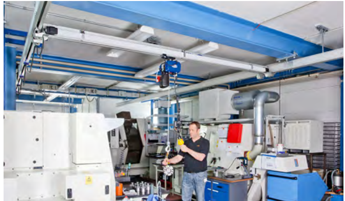
Low ceiling mounted aluminum single bridge crane system with conductor line to accommodate the low ceiling height
