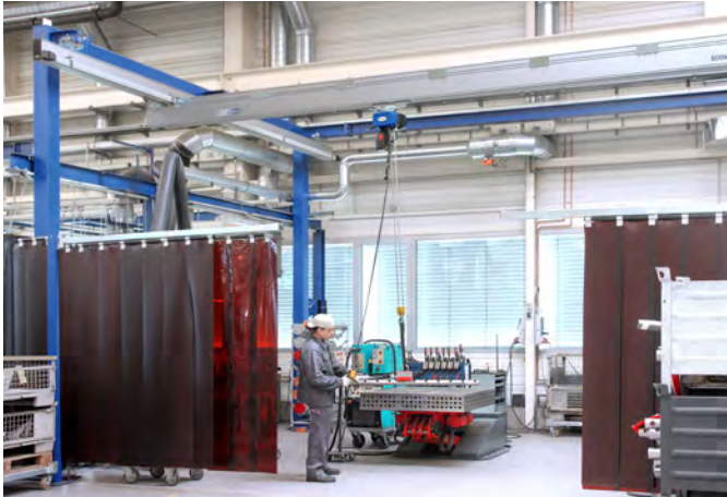
Aluminum single bridge crane system with reinforced section and a conductor line used with a chain hoist and a magnet
