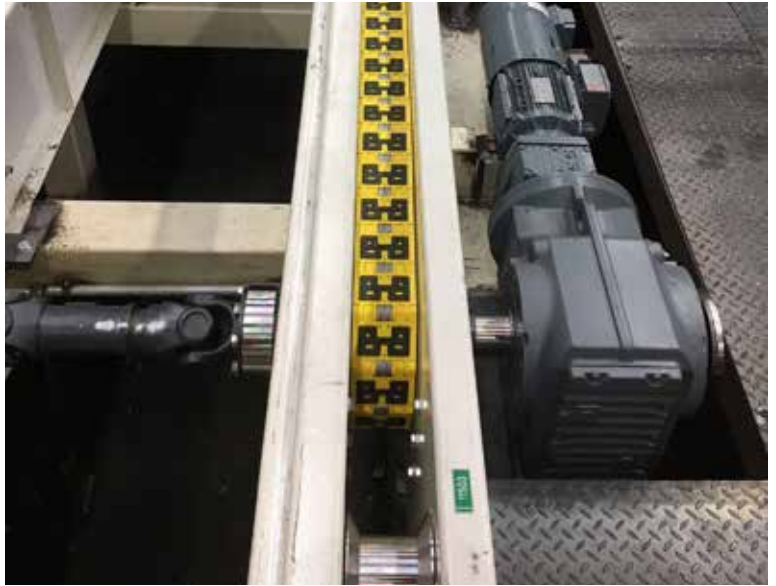
Conveyor equipped with Rexnord 3125 HYB 12 Series MatTop Chain.
